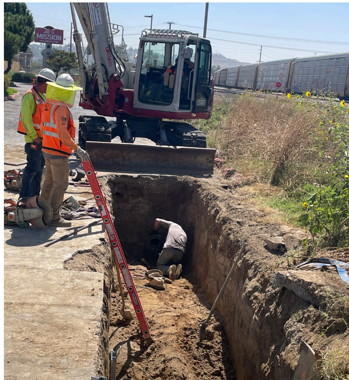
Crews performing utility line relocation work in the Felspar St. western business plaza.
