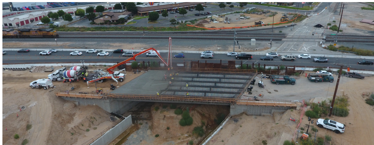
Project Milestone: Crews placing concrete on the Van Buren Boulevard Bridge deck.
