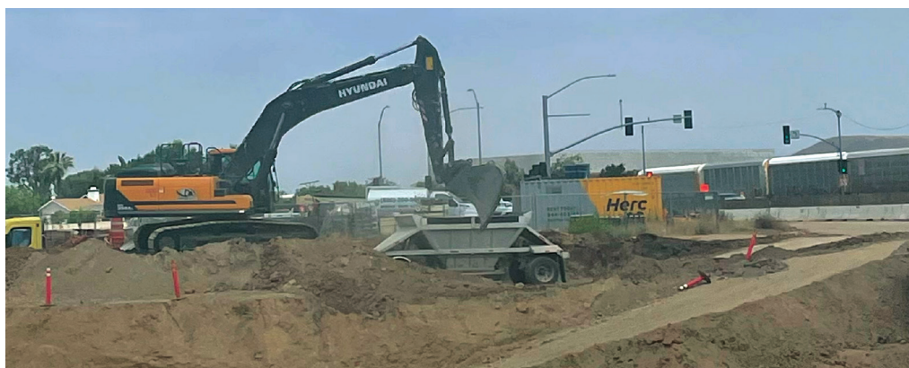
Crews moving dirt in the “main yard”, behind the Jurupa Road Underpass system.
